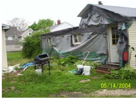
Before – Rear view shows poor condition
