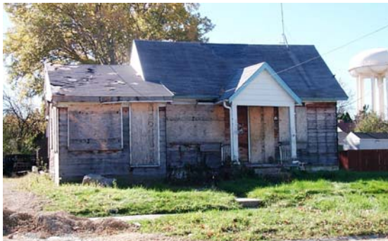
Before – Front view shows the house in poor condition. City assisted with demolition
